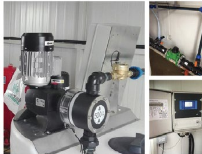
Figure 53. Fertilizer injection calibrated by a dosing pump under the command of the fertigation control unit.
